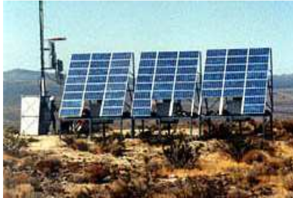
Figure 11: Use of solar power for Telecom System (Coutesy: Kyocera Solar. Inc.)
