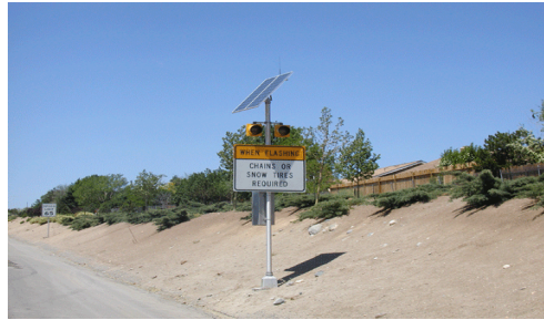
Figure 13: Use of PV unit for traffic signaling (Coutesy: Kyocera Solar, Inc.)
